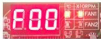
channel 1 stop-rotating temperature
